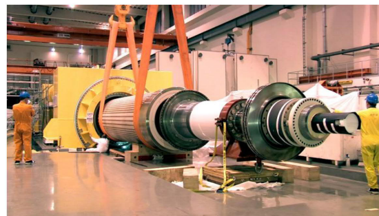
OKG Photo-library. http://www.okg.se/en/Media/Photo-library Noudettu 21.11.2013
